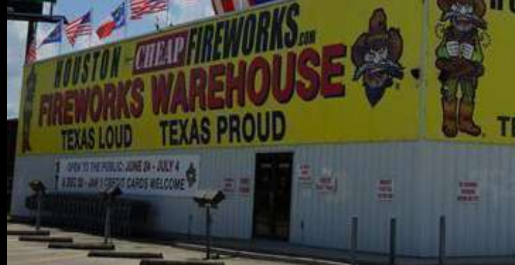
blown up metal fascia clad
